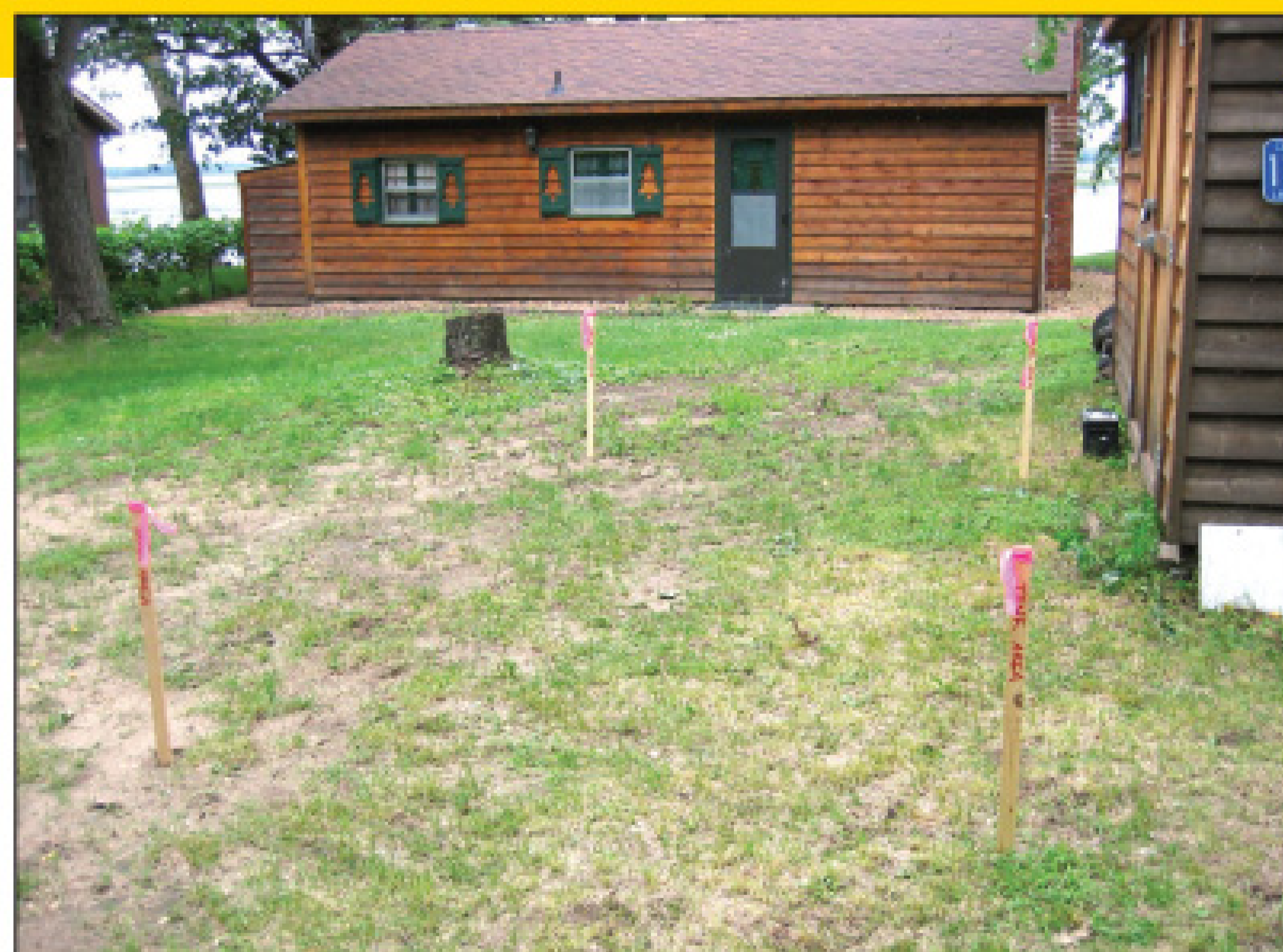
System locations staked in a small lot area. (Photography by Dave Gustafson, P.E.)
