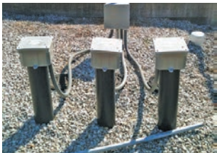
3 Salcor 3G UV Units (Parallel Array) in Extended Aeration
