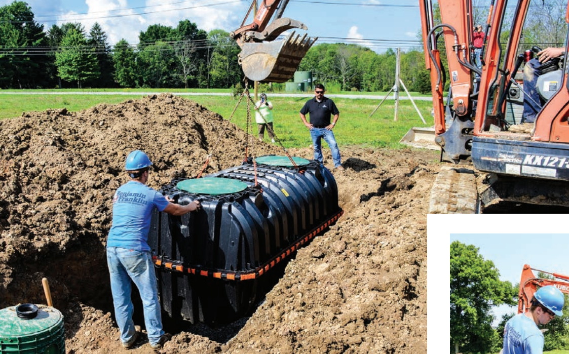
◀ Benjamin Franklin Plumbing employees install an Infiltrator Water Technologies IM-1060 tank behind a Jet Inc. treatment tank.
