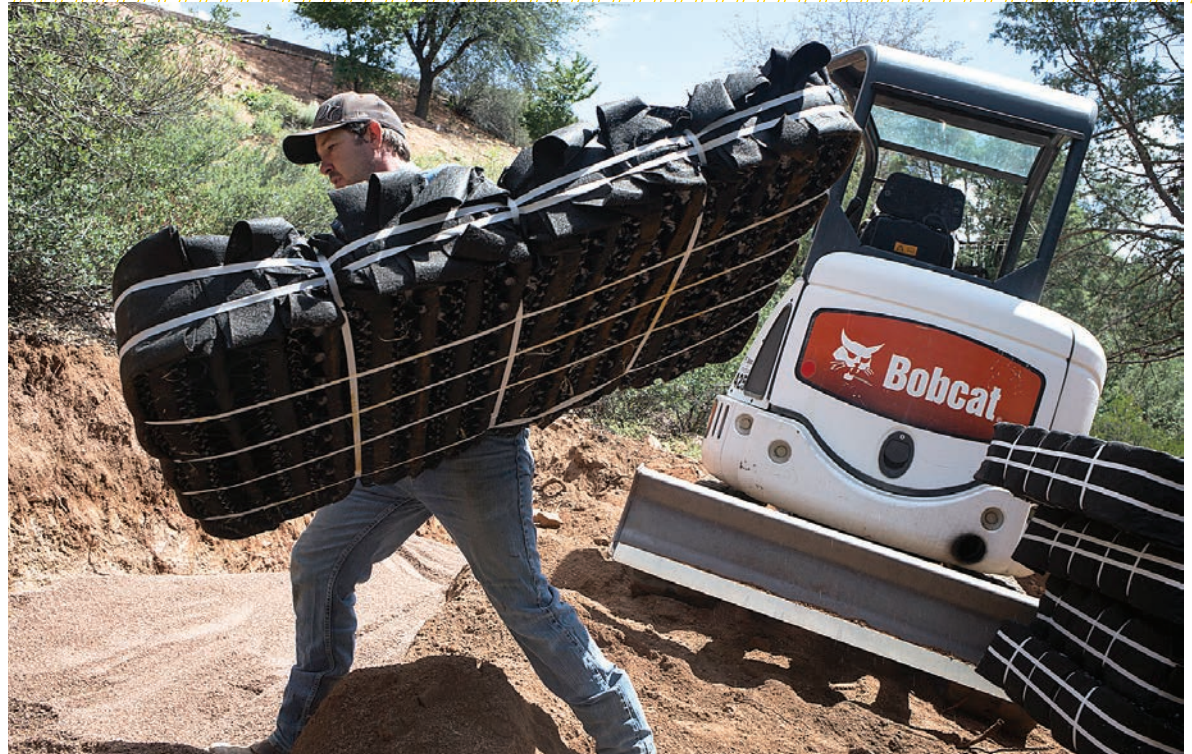
▲ Willie Brown usually works by himself on onsite wastewater jobs. That means hauling around his own supplies, in this case 3-by-4-foot Eljen GSF, or Geotextile Sand Filter, drainfield media. His Bobcat excavator is shown in the background.
