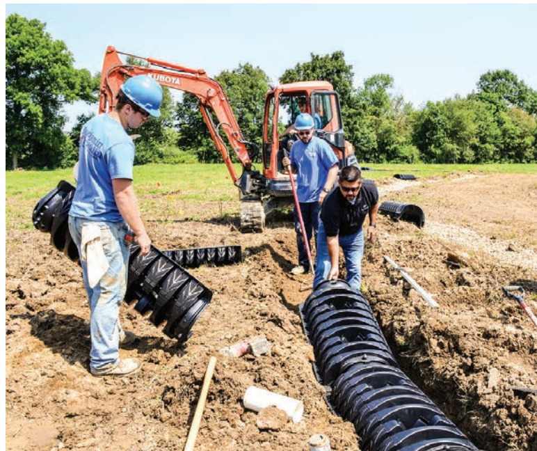
▼ Zak Sherman, of Infiltrator Water Technologies, demonstrates installation of Quick4 low-profile chambers. Also pictured are workers from the DeBord/Benjamin Franklin Plumbing installation team.
