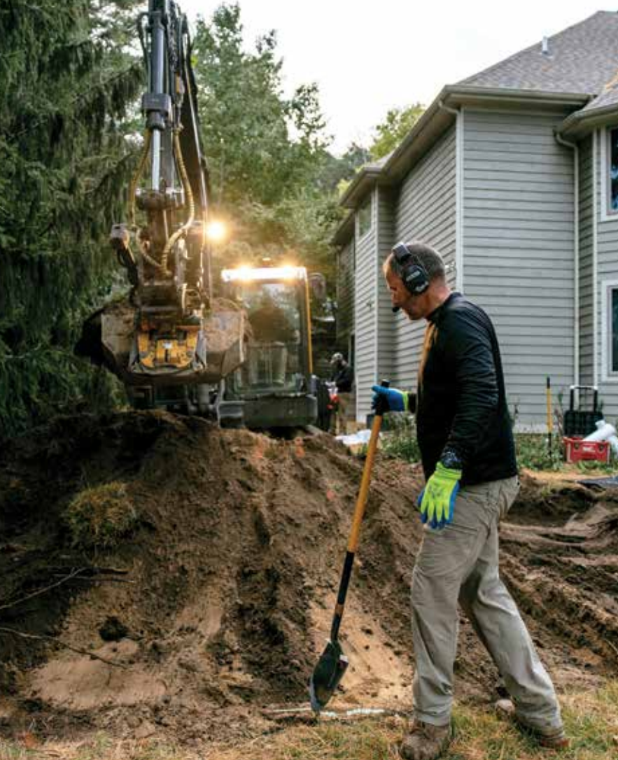
◀ Ethan Vanderwarf operates the excavator while Travis Gemmell locates the drain area.
