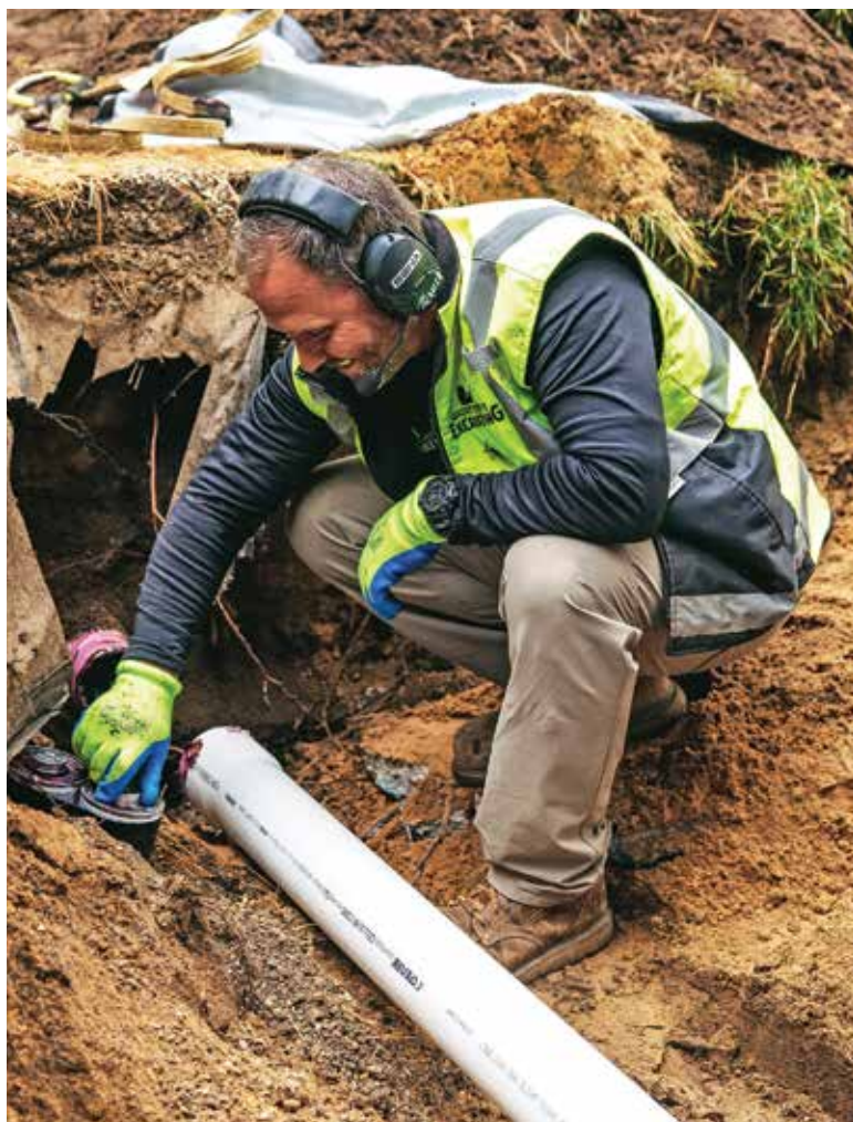
▲ Gemmell and his crew rely frequently on Sena headsets for both ear protection and communication. They keep them talking and safe even when their hands are full installing pipe. (Photography by Lucian Witmer)
